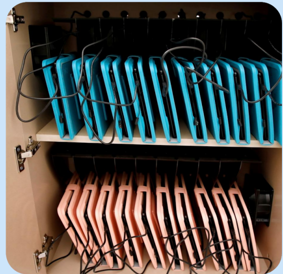
Cables Passed to Charging Compartment
